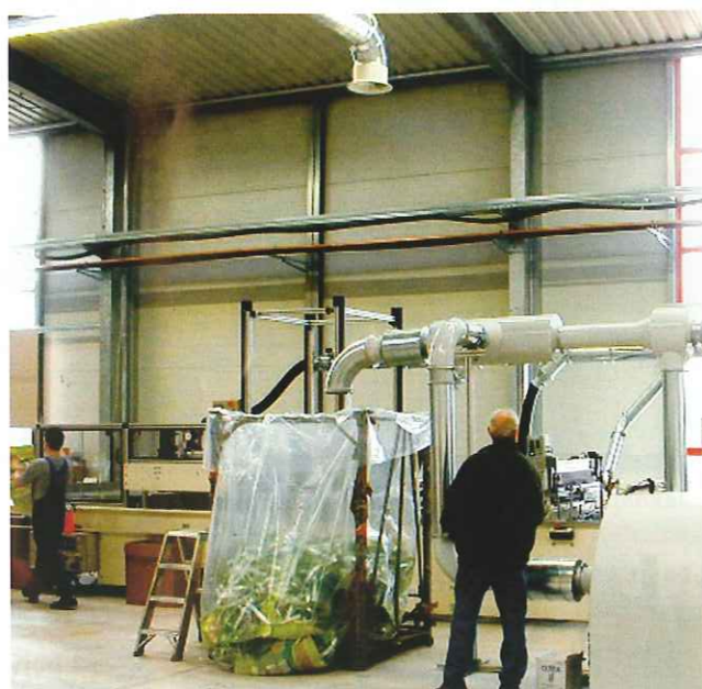
In the original installation the edge trims were collected in big bags
