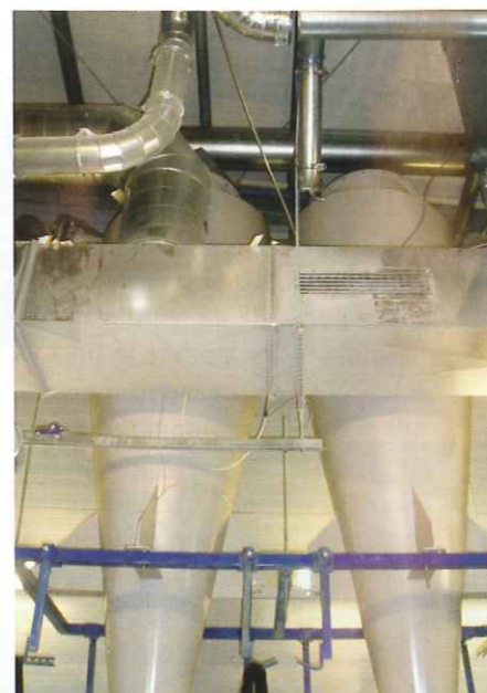
The modern vacuum extraction unit
