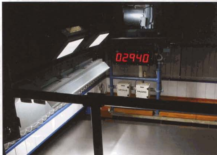
A typical finishing line system arrangement with the Q-eye high resolution video inspection system
